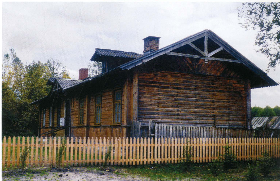
13. Dom kolejarski podczas remontu. Fot. D. Stankiewicz, 2014. Railwaymen's house during renovation. Photo: D. Stankiewicz, 2014.
