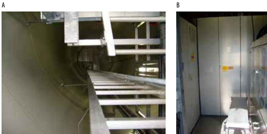
Fig. 3.19. The interior of a tubular steel tower A) service ladder, B) control cabinet (Source: photos by T.J. Teleszewski)
