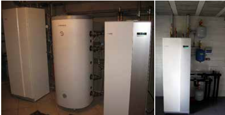
Fig. 5.27. Examples of ground heat pumps in buildings (Source: Smuczyńska, 2015)
