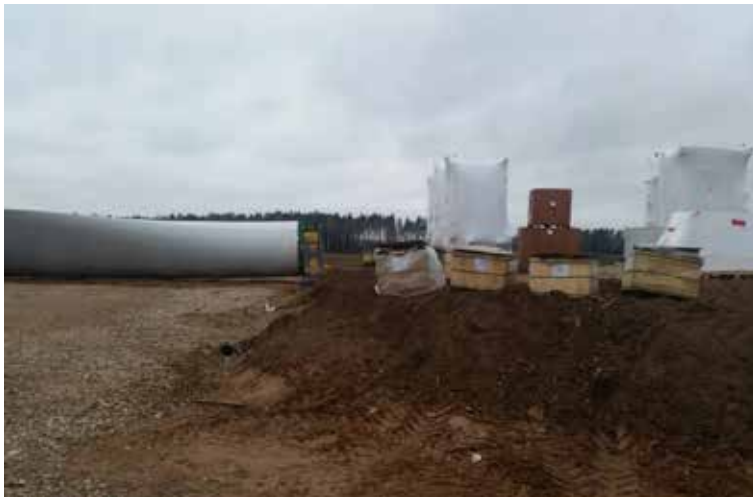
Fig. 3.11. During the construction of a wind turbine, it is necessary to ensure safe storage of expensive equipment (Source: photo by K. Jasiūnas)
