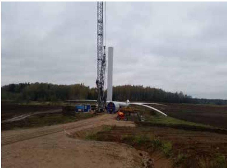
Fig. 3.13. Installation of wind turbine elements in a field (Source: photo by K. Jasiūnas)
