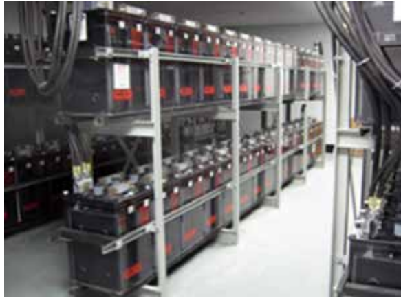
Fig. 8.5. UPS image (Source: WEB-2)
