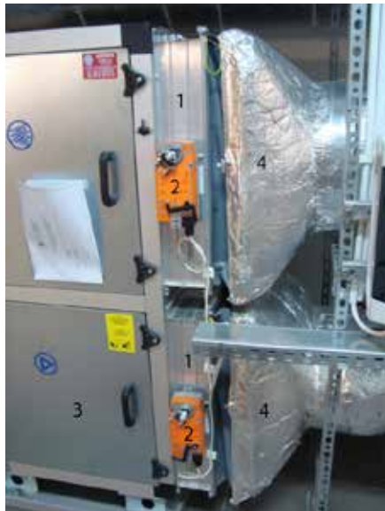
Fig. 8.13. An example of application of a throttle regulation: 1 – an air damper, 2 – an electric actuator, 3 – a fan, 4 – a ventilation duct (Source: T.J. Teleszewski's private archive)
