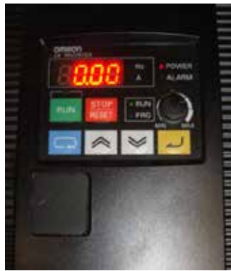
Fig. 8.12. A frequency converter control panel (Source: T.J. Teleszewski's private archive)
