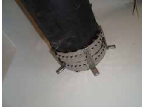
Fig. 8.19. Intumescent pipe collars (Source: photo by T.J. Teleszewski)
