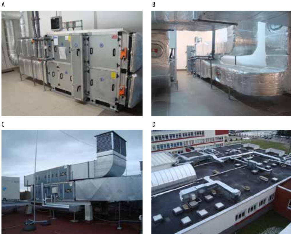
Fig. 8.5. Location of the AHU: A-B) in the basement, C-D) on the roof (Source: photos by T.J. Teleszewski)
