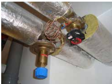
Fig. 7.15. An example of a direct-operated pressure regulator installed on a central heating system (Source: T.J.Teleszewski's private archive)
