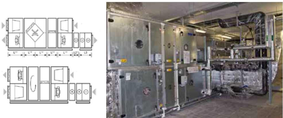
Fig. 8.4. AHU construction (Source: R. Bilinskienė's private archive; WEB-1,3)
