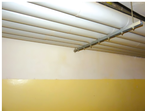
FIG. 7.13. View of six individual heating pipes in the analyzed example (Source: photo by T. Telaszewski)
