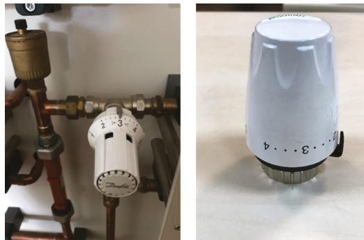
FIG. 2.18. Thermostatic valves (Source: photo by R. Bilinskiene)
