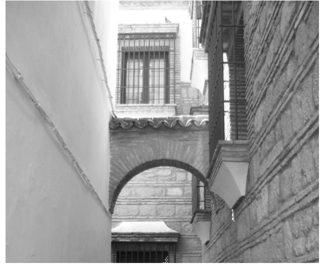
Fig. 5. The conductors on the façade in Cordoba (photo K. Gładyszewska-Fiedoruk).
